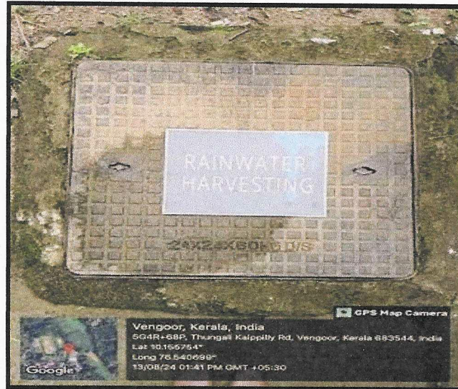
Underground Rainwater Harvesting Pit
