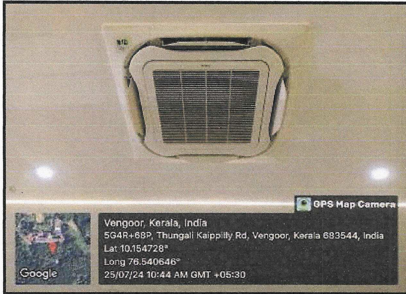
Air Conditioner in the Board Room
