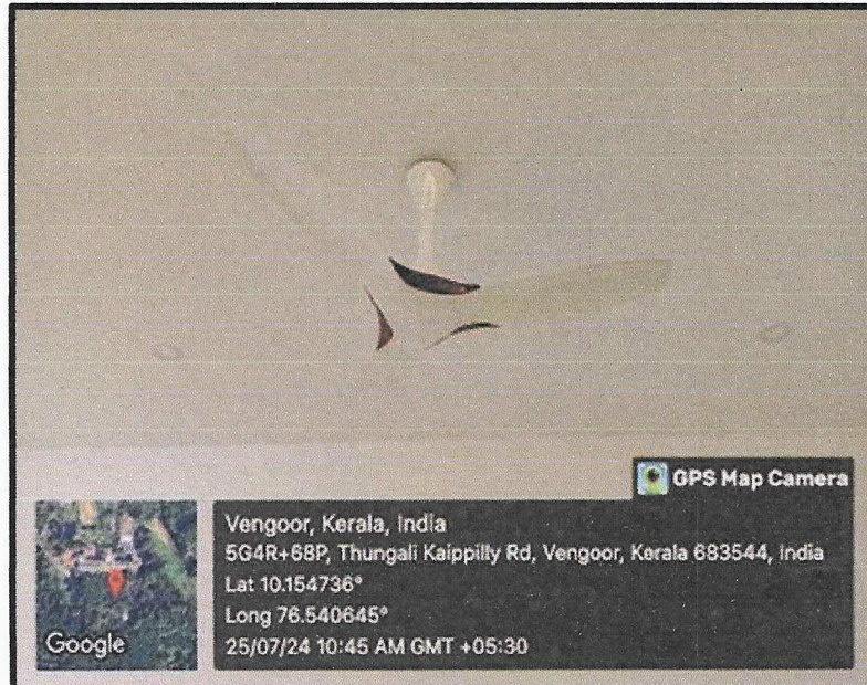
Smart Fan in the Board Room
