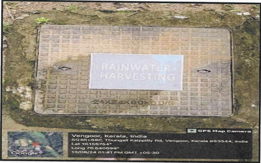
Underground Rainwater Harvesting Pit
