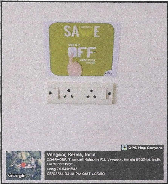
"Save Energy": Posters Above Switch Boards
