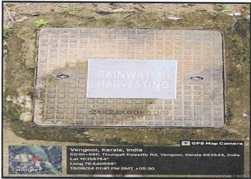
Underground Storage Pit of Rainwater Harvesting System
