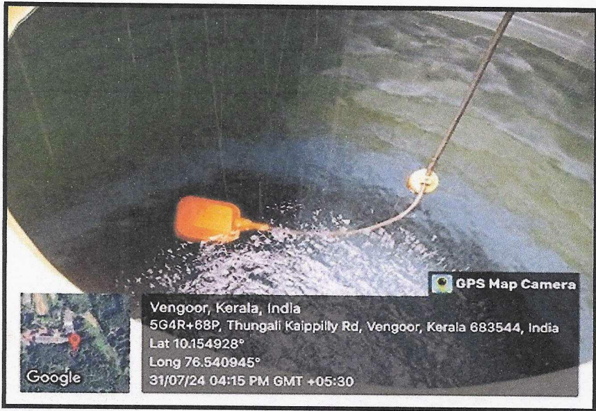
A Floating Valve inside the Water Tank
