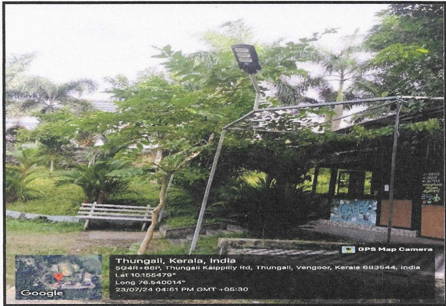
Street Light Located Near the Cafeteria
