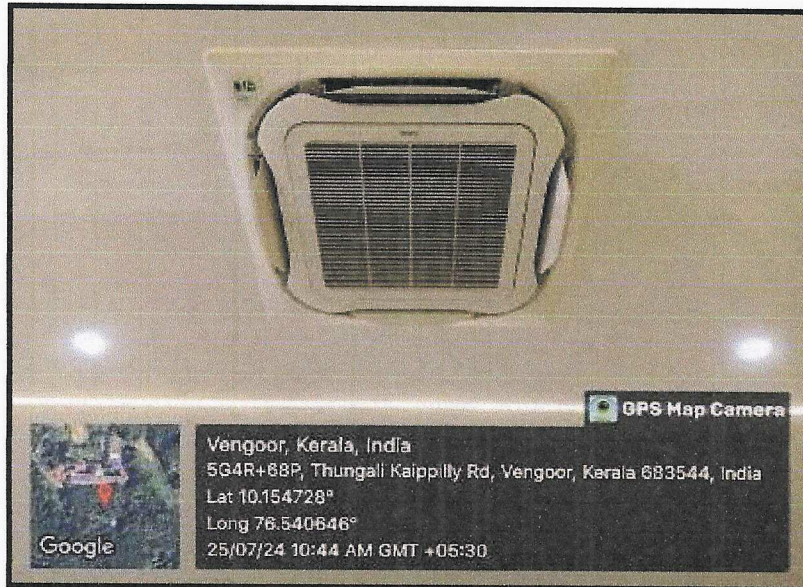
Air Conditioner in the Board Room
