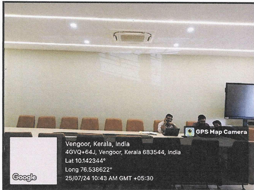
LED Lights Illuminating RVCAS Board Room
