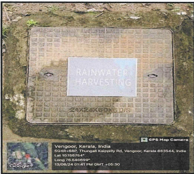
Underground Rainwater Harvesting Pit
