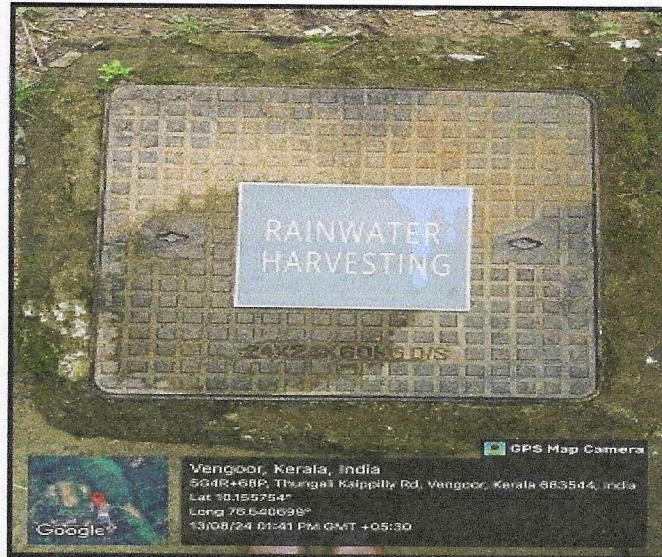
Underground Rainwater Harvesting Pit
