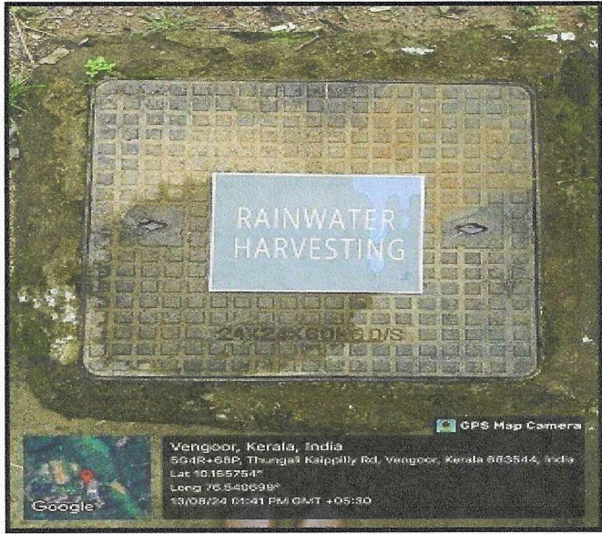
Underground Rainwater Harvesting Pit
