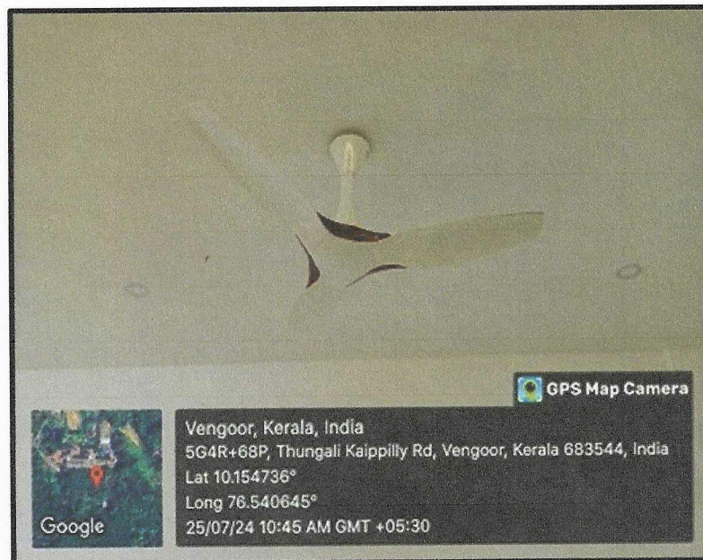
Smart Fan in the Board Room
