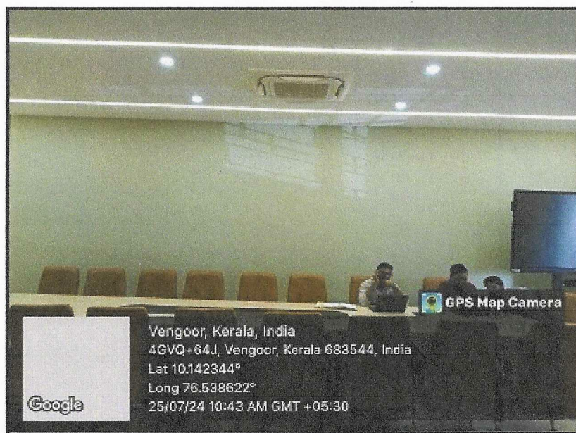
LED Lights Illuminating RVCAS Board Room
