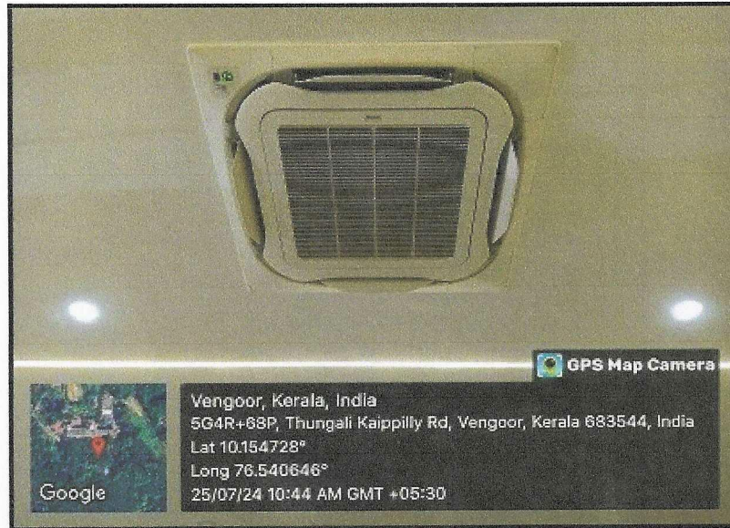
Air Conditioner in the Board Room
