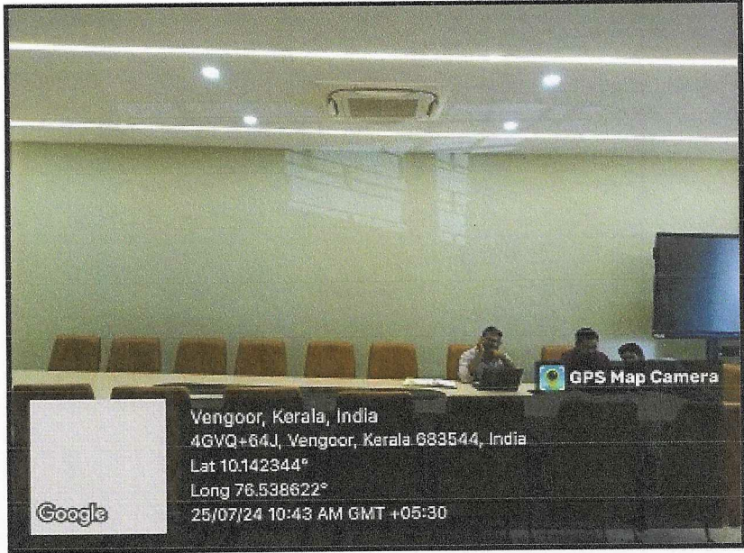
LED Lights Illuminating RVCAS Board Room
