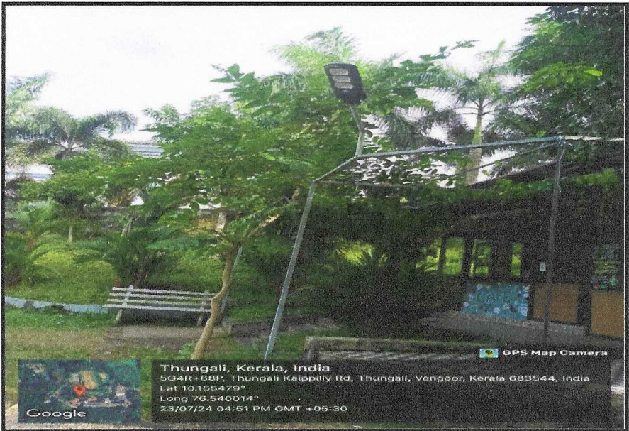
Street Light Located Near the Cafeteria
