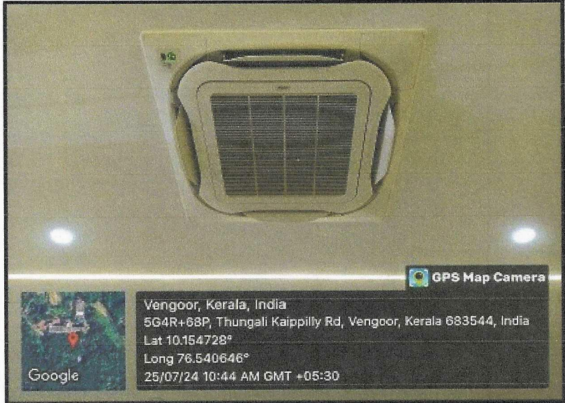
Air Conditioner in the Board Room
