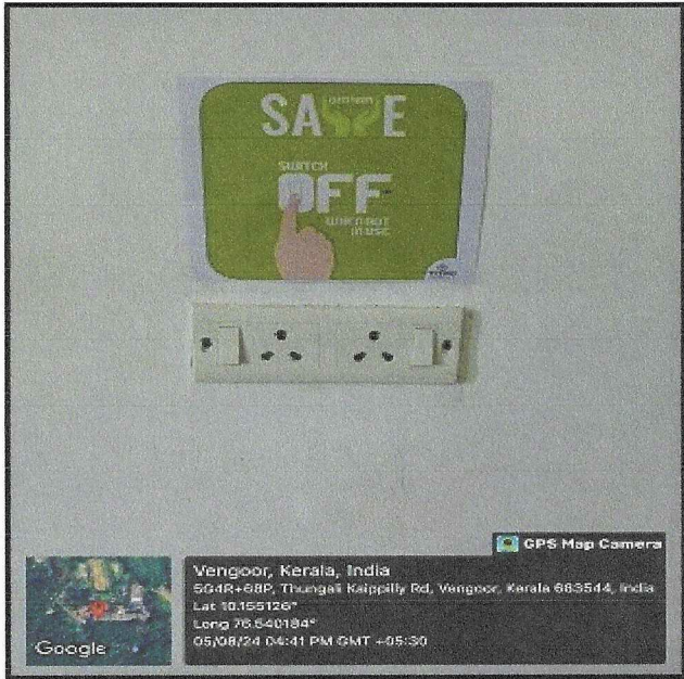
“Save Energy”: Posters Above Switch Boards
