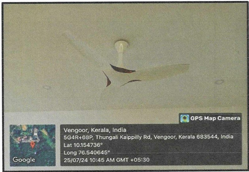
Smart Fan in the Board Room
