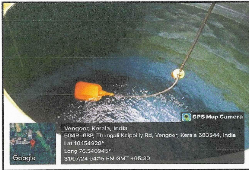
A Floating Valve inside the Water Tank
