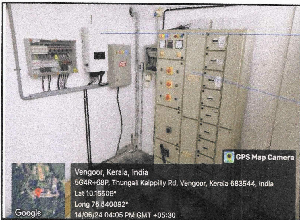
Electricity Control Room
